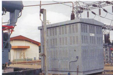
Neutral earthing resistor (Indonesia), 24 KV - 1150 A - 10 sec.
