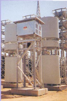
Harmonic filter resistor Manitoba (Canada)
