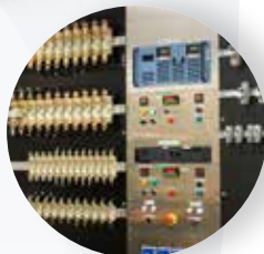
Electrical performance Test Lab
