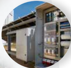
Pv Solar Test Lab
