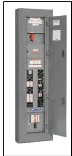
Figure 6— Mersen Fused Coordination Panelboard
