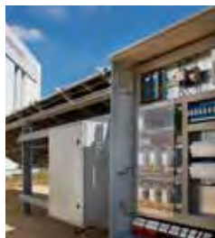
Pv Solar Test Lab
